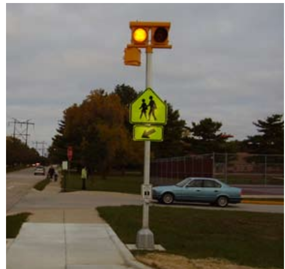
Flashing signals installed in 2009 at Cumberland Elementary School. Source: HWC
